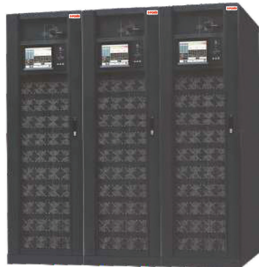
Three units in parallel
